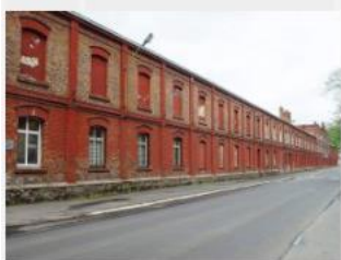
Factory building in Kraslice, 2007 (Photo: Flossenbürg Concentration Camp Memorial). A textile factory, located in one section of the long complex, is once again operating today.
